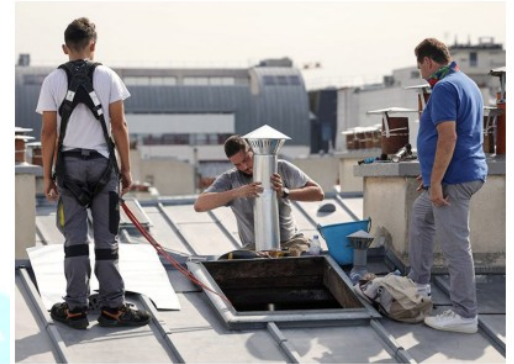
In process: A roofer and zinc worker on the roof of a building in Paris. AFP
