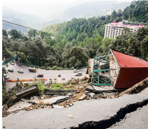
A road damaged by a landslide triggered by heavy rain at Balugani in Shimla on August 21. Most regions of India now expect weather extremes in all seasons. PTI
