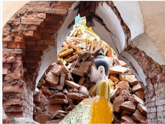
Mass destruction: A damaged pagoda in the aftermath of the earthquake in Amarapura township, Mandalay, Myanmar, on April 2, 2025.
